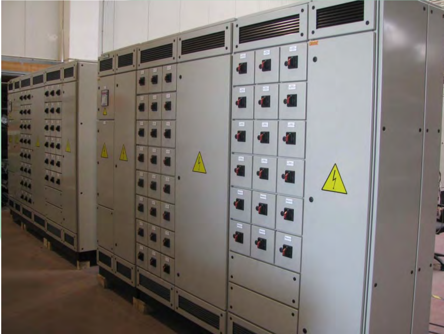
Draw-out panels in “power cassette version” (Elsteel panel system, ABB components)
