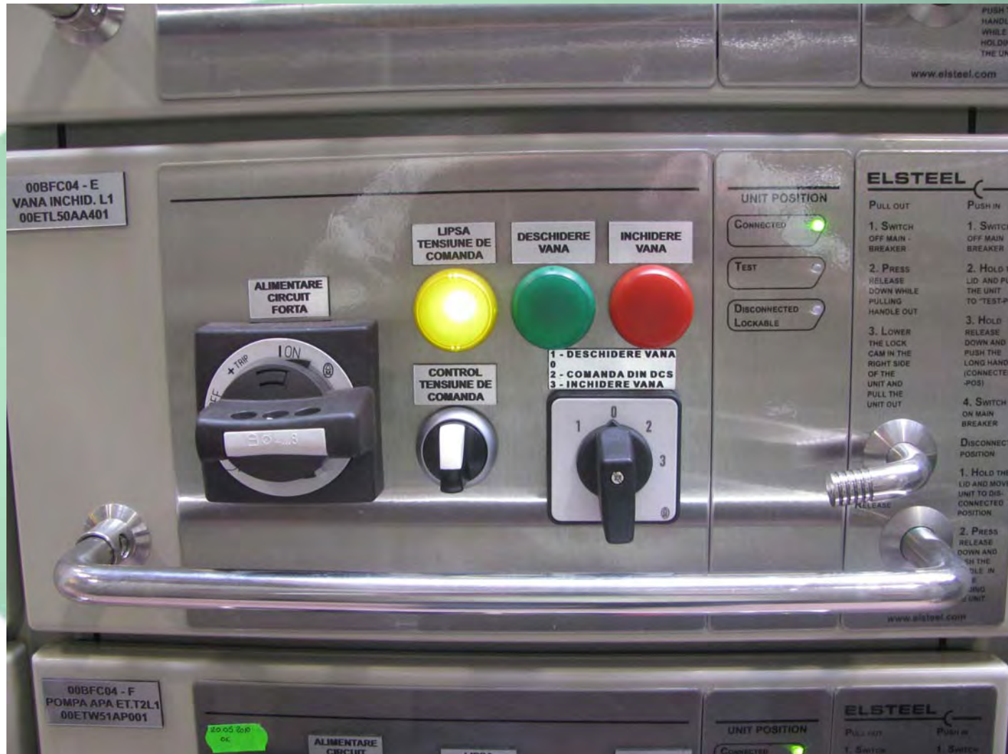
Draw-out technology (Elsteel panel system, with Eaton components)
