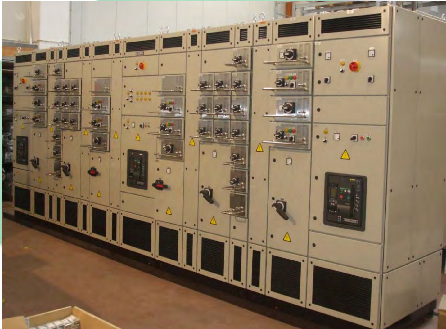
Panel for Compressed Air Station (Elsteel panel system, with Eaton components)
